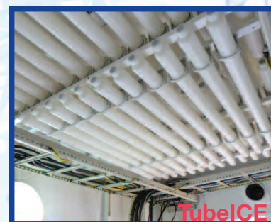
Typical Telecom Shelter Passive Cooling
